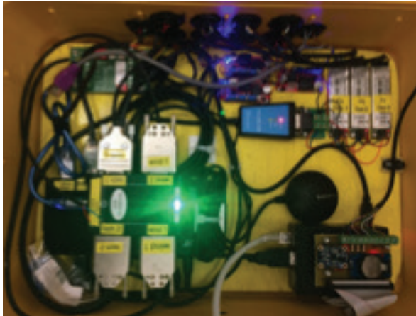
Figure 9. Data acquisition system in pelicase box.
