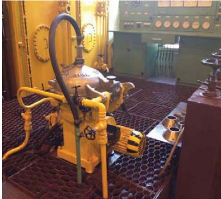
Figure 1. Fuel centrifuge Alfa Laval.
