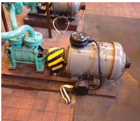
Figure 3. Outboard water pump.
