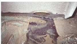
Figure 3. Sediments accumulate in ballast water tanks in areas with flow stagnation.
